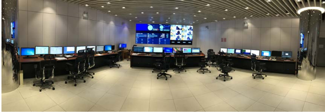
Figure 1.1 Layout of Central Control Room
